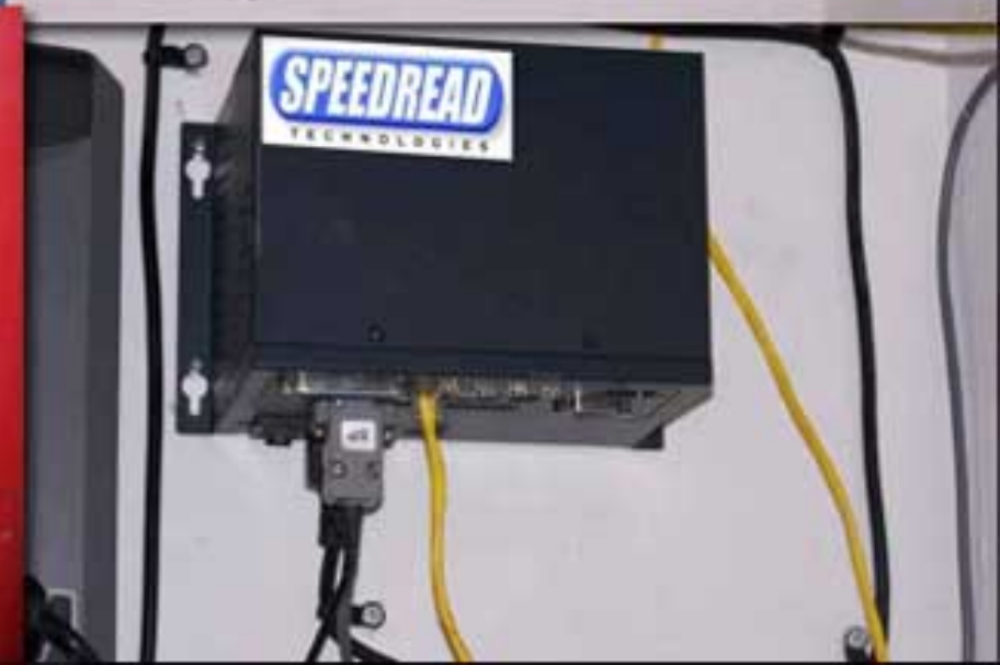
2" Hersey Meter, Cooling Tower Make Up Water, Neiman Marcus
